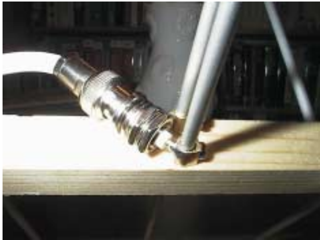
Feed point close-up
